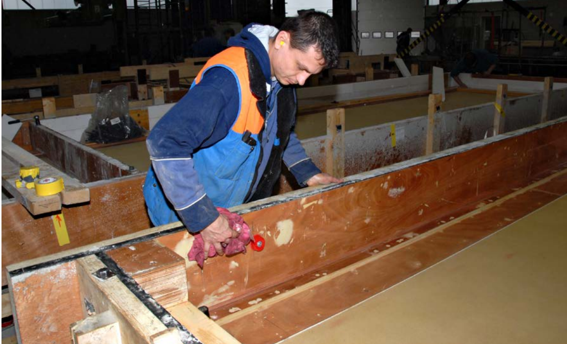
The concrete mould is being cleaned prior to the next concrete casting.
